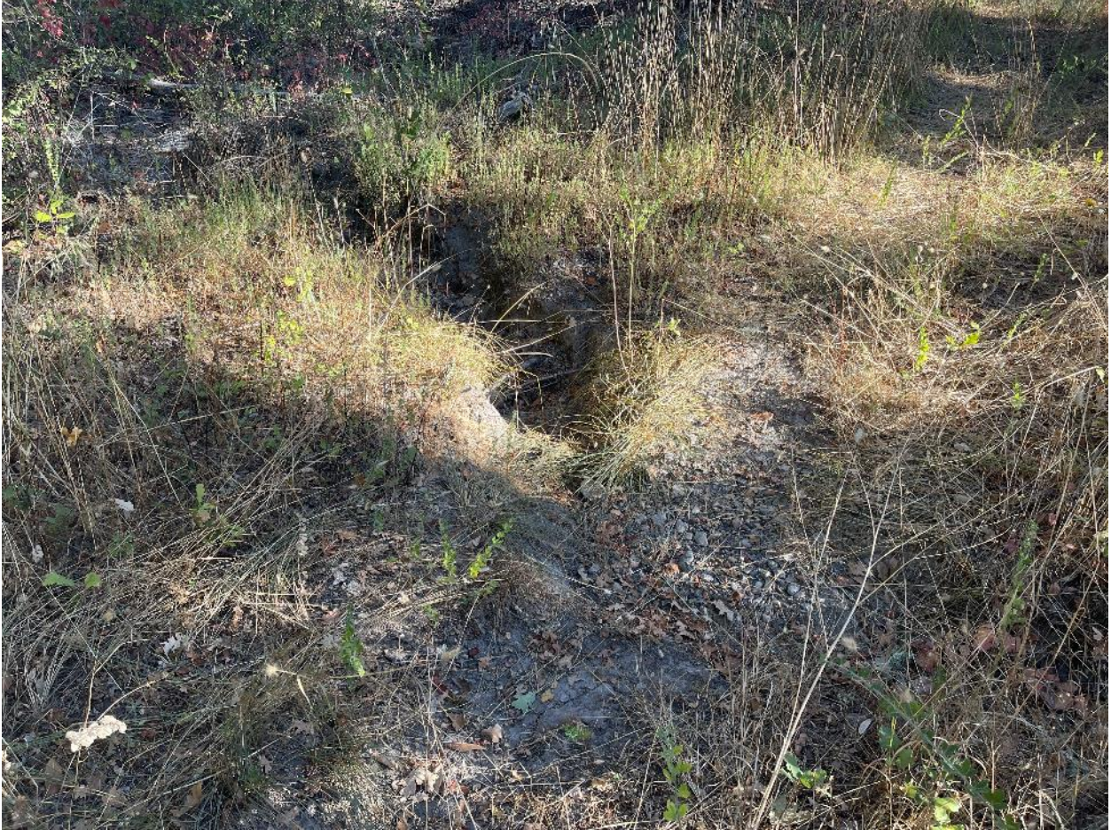
Figure 47: Chronic Erosion Site #6, Headcutting across fire service road as a result of concentrated flow running down middle of road from steeper sections uphill.
