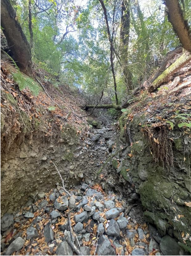
Figure 11. Retention Opportunity #3, sluice canyon exit with headcut visible.
