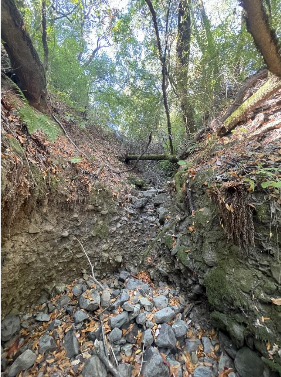
Figure 44: Chronic Erosion Site #5, Headcut at Sluice canyon outlet. Erosion occurs all throughout this canyon, at this outlet and further down between there and Asbury Creek.
