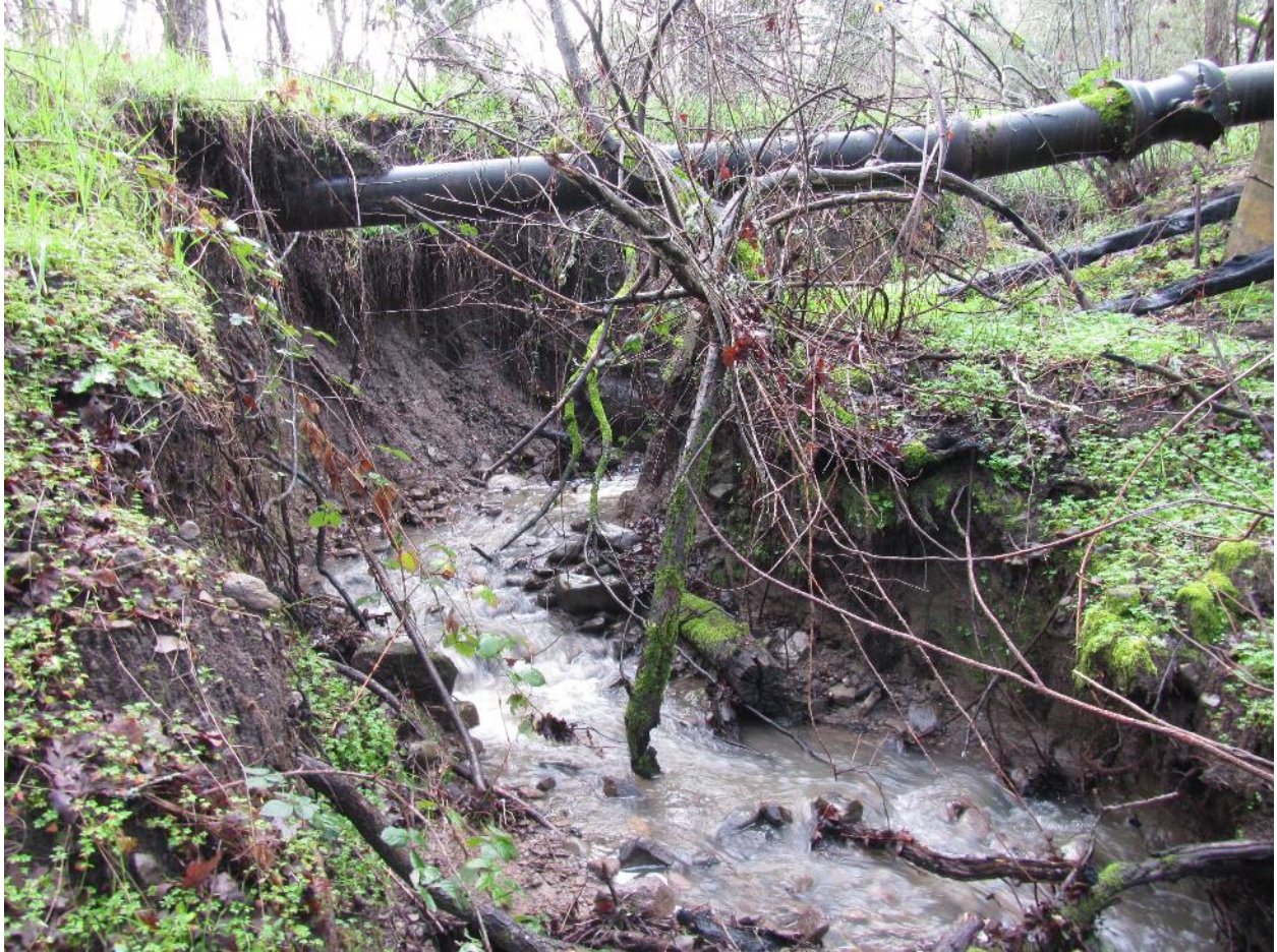
Figure 40: Chronic Erosion Site #1 Extensive culvert-related gully formation at lower Corridor Creek South. A large diameter conveyance pipeline connecting Fern Lake and Lake Suttonfield is threatened with breach at this location.
