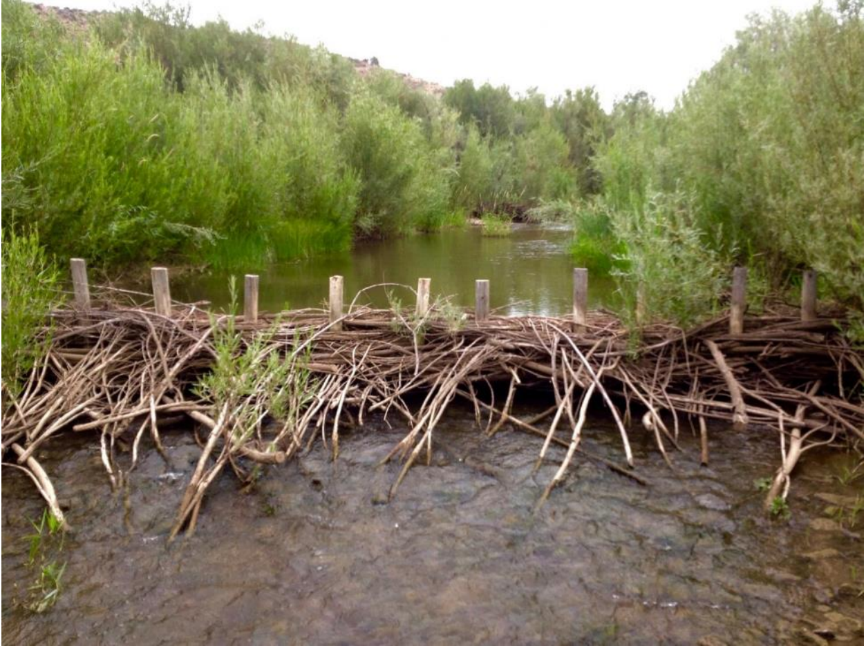
Figure 24: Example of Beaver Dam Analog (BDA) allowing for water retention in a low slope drainage area..
