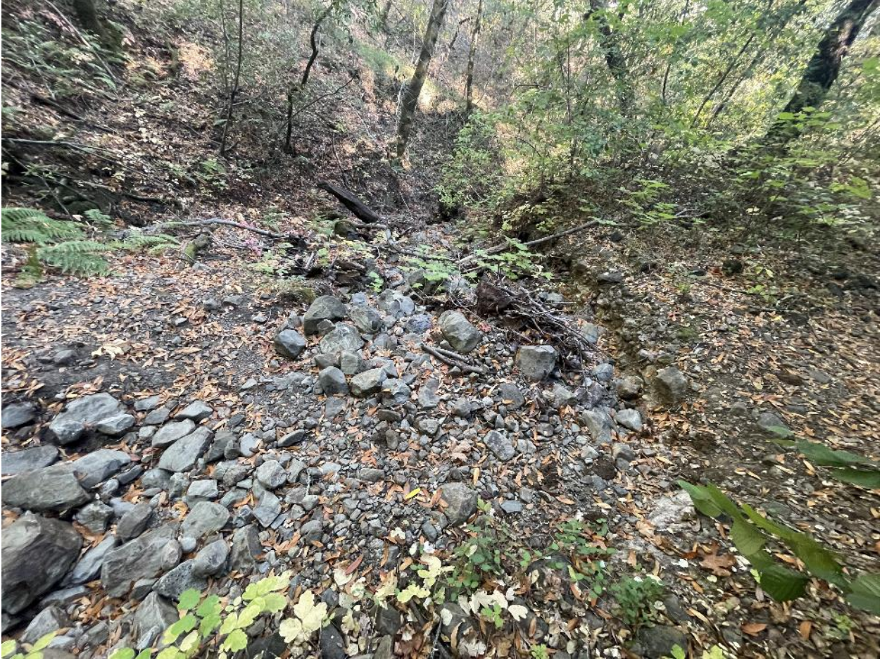
Figure 45: Chronic Erosion Site #5, Wash across fire service road shown along with additional erosive area further below that.
