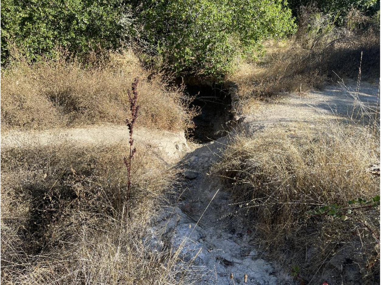
Figure 14: Chronic Erosion Site #4, Headcut on constructed Fern Lake overflow channel impacting fire service road. Road is currently impassable by emergency vehicles.
