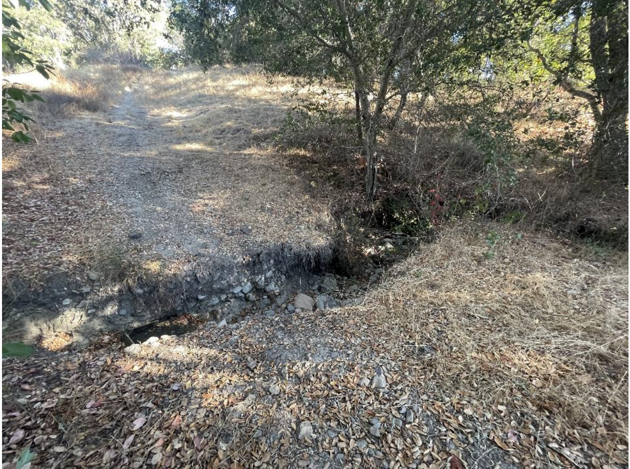
Figure 17. Water Retention Opportunity #4 Headcutting section of Corridor Creek North just upstream of the tributary branch point. A fire service road has become impassable at this location.
